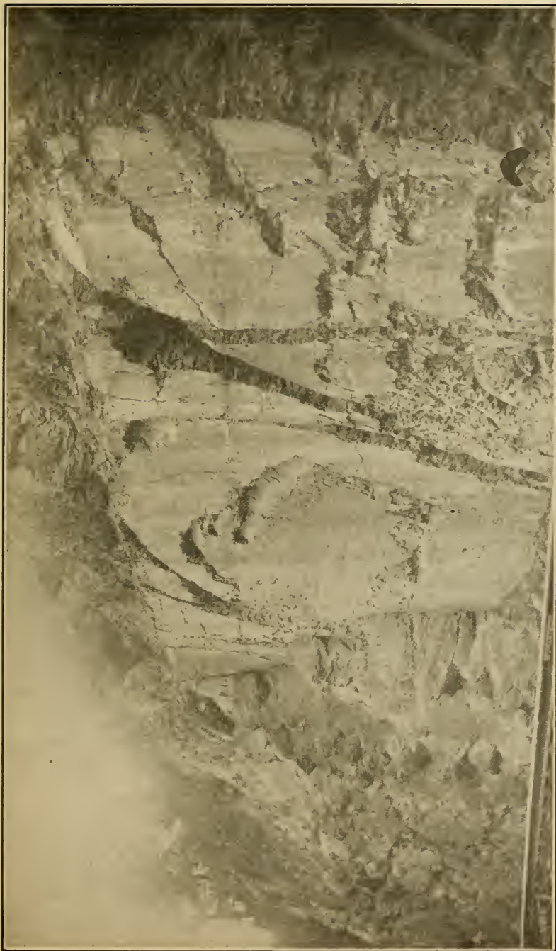
PLATE XXIII.—A joint-plane in Marcellus strata along which somewhat of faulting has taken place. The slickensided surface has weathered off in places. The direction of the fault is N. 73° E. The location is in the third cut west of Oldtown, Maryland, opposite the flat at Greenspring.
